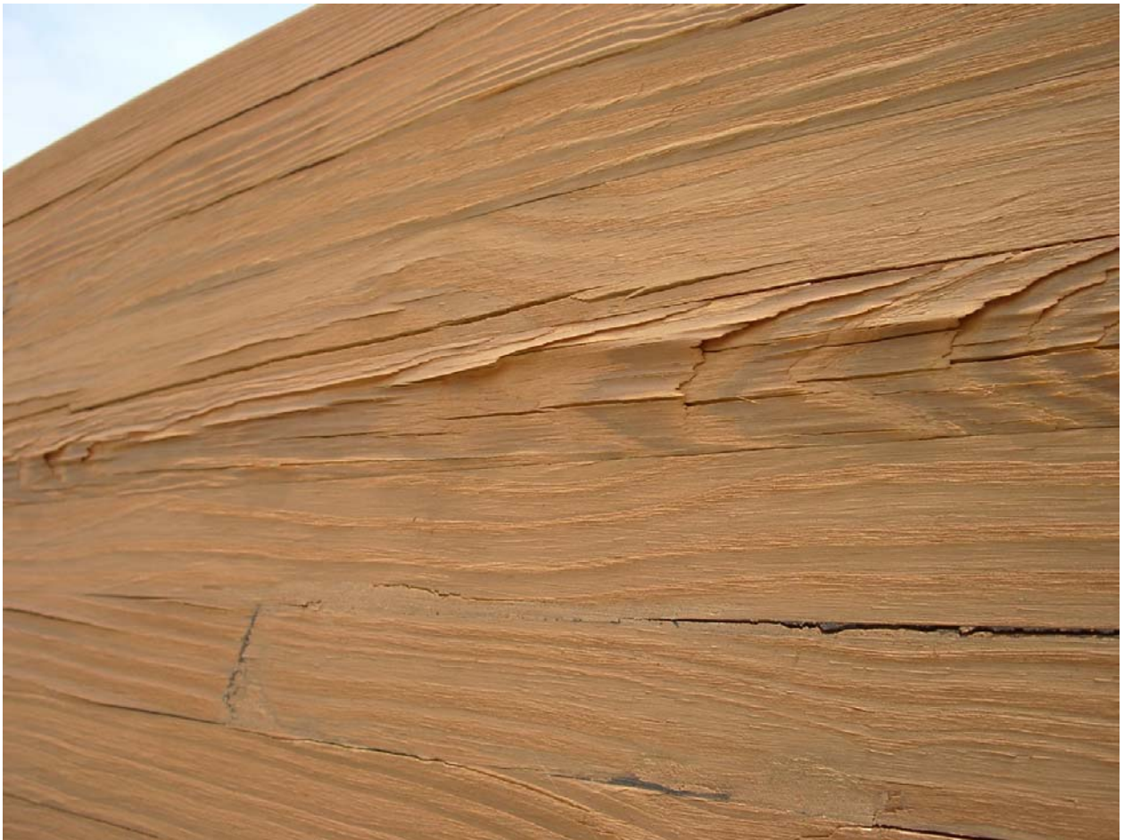
Figure 2. Raised grain, shelling, and checking in glulam beam treated with CCA after bonding.
